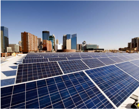
Rooftop solar panels
