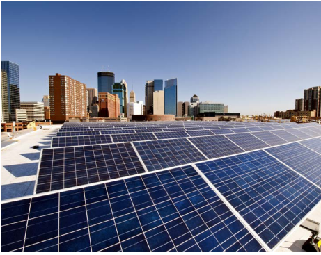
Rooftop solar panels
